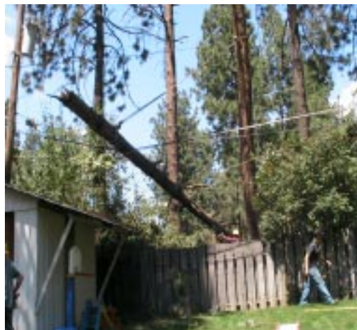
Example of downed power lines along back lot lines in the District as a result of the storm
