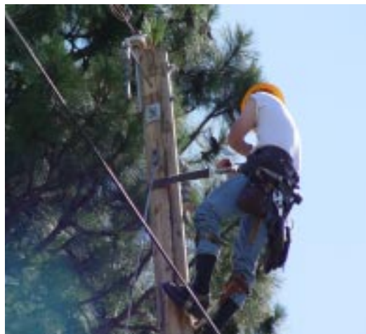
Vera Linemen working on damage to overhead lines
